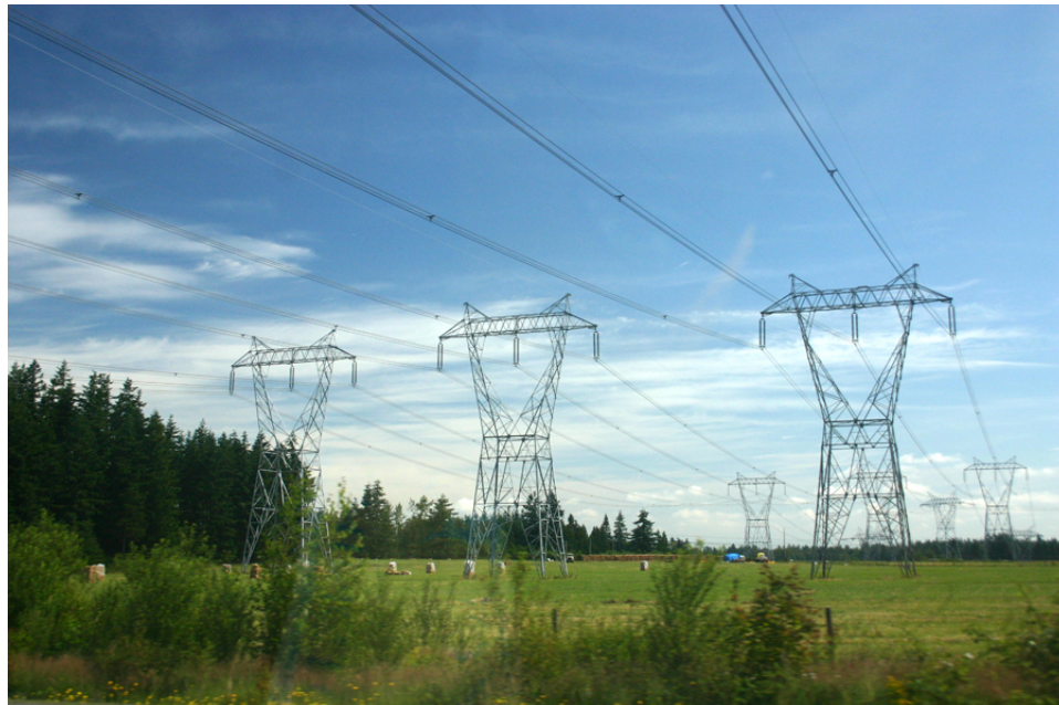
Three-phase power distribution lines.
